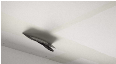
Once the first coat is dry, apply a layer of Ready-Mix Filler (use a 240mm wide knife).
