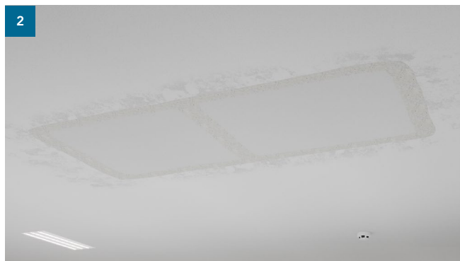
Installing new panels and filling edges. Cut a matching "plug" out of a new Rockfon Mono Acoustic panel and fasten the "plug" in the hole using the filler.
